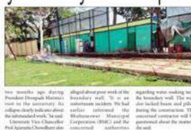
Substandard work during Prez visit alleged. A large portion of the boundary wall of the Rama Devi Women's University here collapsed on Sunday.
